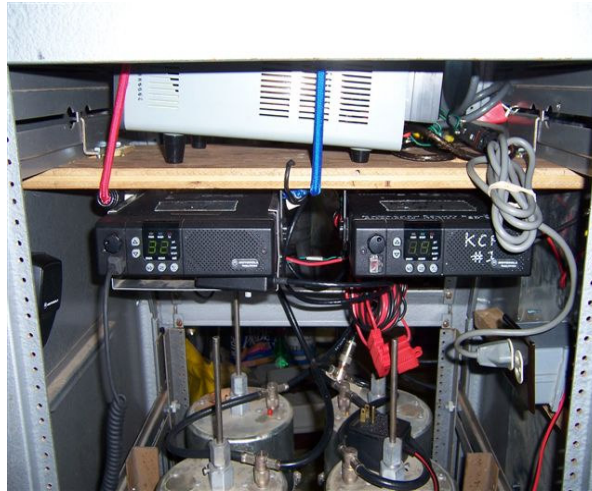
KCRA's new Portable Repeater
